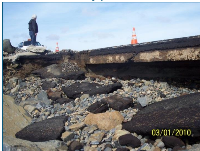
Wave-induced Undermining of HWY 101
