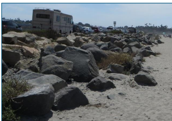
Revetment in Fair Condition
