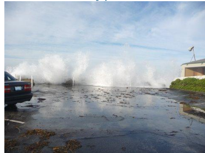
Wave Attack on Revetment Fronting Restaurant Row
