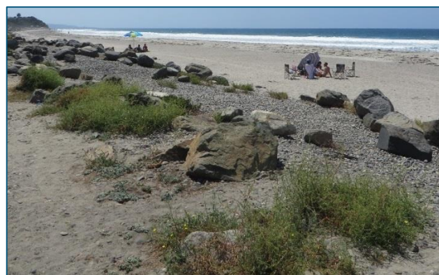
Revetment in Poor Condition
